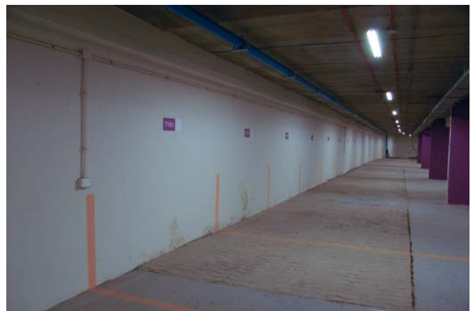
Figure 1 Level -7 Basement Wall of Torre Titanium La Portada in Santiago, Chile after February 27, 2010 earthquake
